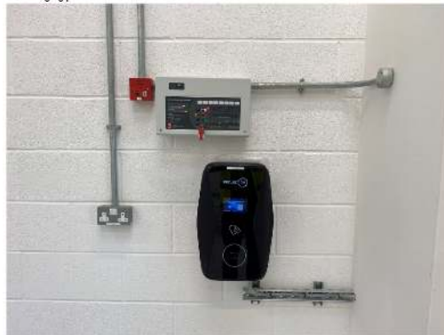
Car Charging point
